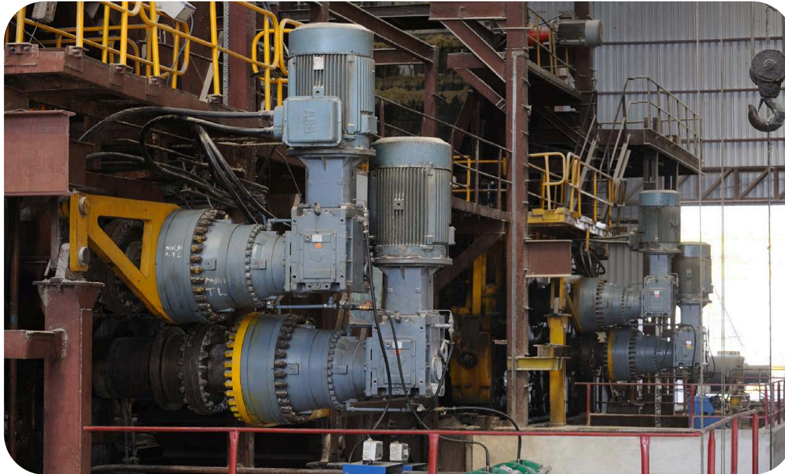
Fig: Actual installation at Jay Mahesh Site, India
